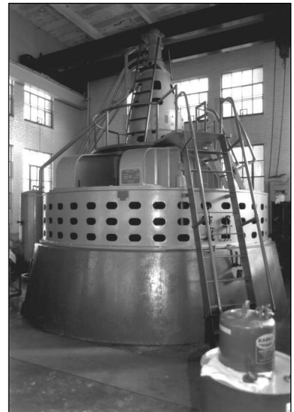
The powerhouse contains a single generating unit, an 800kw alternator made by the Electric Machine Manufacturing Company of Minneapolis.
