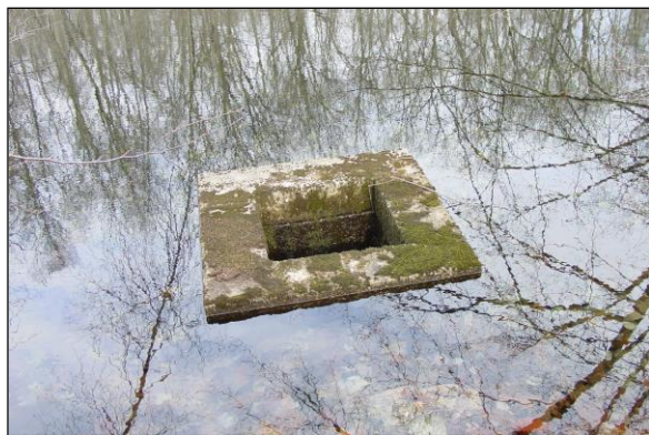
Gravity reservoir outflow structure.
