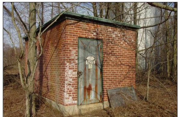
Typical deep-well pump house.
