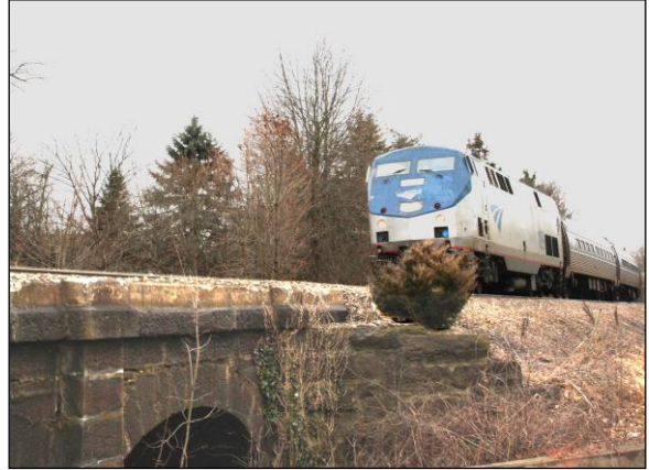
Many of the bridges along the corridor are stone arches, such as this 1870 example in Berlin.
