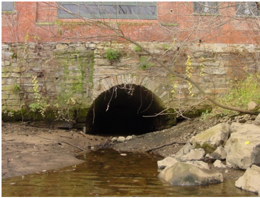
Tailrace arch in a retaining wall along the Housatonic River at low tide within the Shelton Canal Industrial District
